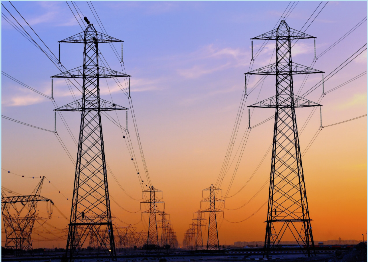
765kV Hyderabad – Wardha D/c line
