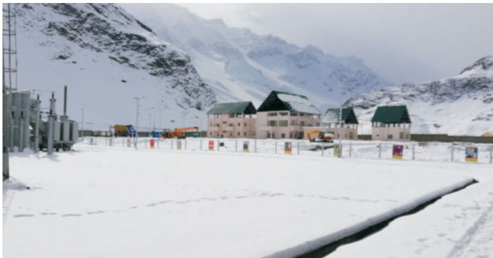
Srinagar-Leh-Kargil-Drass Transmission System
